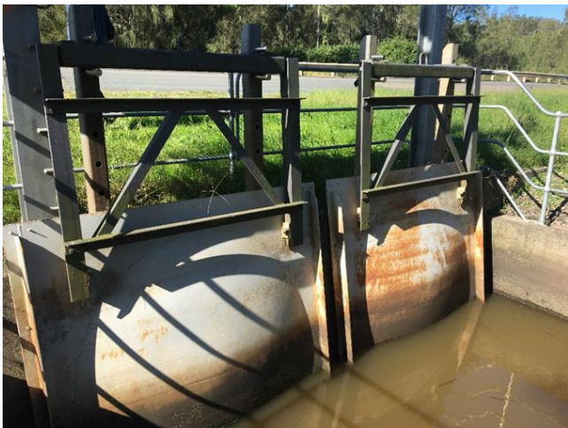
Figure 2-3 Pennington Drain flood gates
